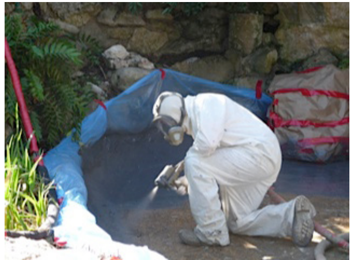
After carefully wrapping stones, pulling plants back, and masking edges by volunteers and park staff, the contractor finally had a dry day to apply the spray liner Photo by Edward Parken for the Taniguchi Garden
